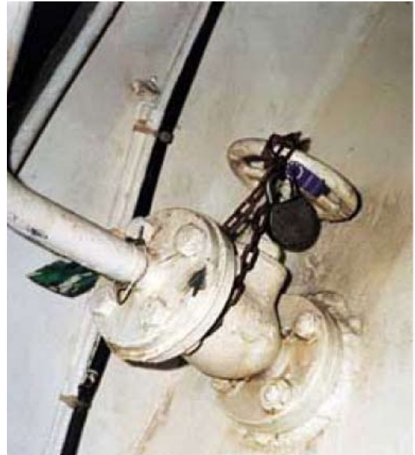
Overboard line for cleaned bilge water from the oily water separator. The hand wheel has been chain locked by the vessel's Chief Engineer at the request of port State control authorities. A seal has also been fitted to the chain.
