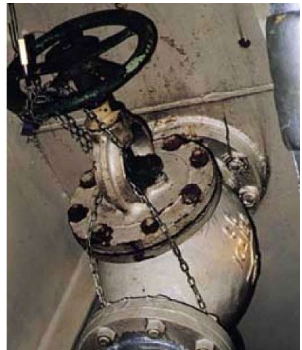
Overboard valve for main bilge/ballast line. The hand wheel has been fitted with a chain and padlock at the request of the port authorities. This is not a good practice as the vessel's bilge pumping system is no longer readily operational.
