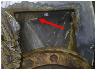
Cracks on water drain outlet (viewed from outside) with signs of leakage
