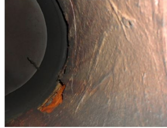
Protective coating inside disch. pipe flaking off at flange
