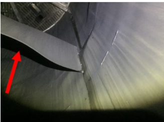
Deformed plates and buckled scrubber housing
